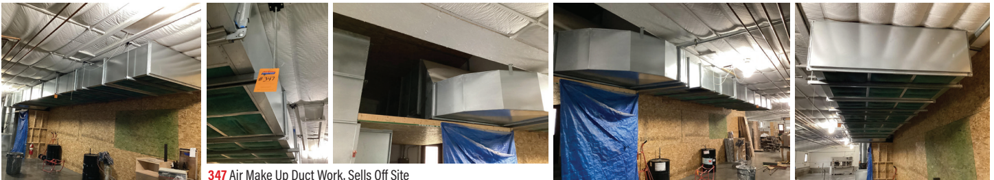
347 Air Make Up Duct Work. Sells Off Site
