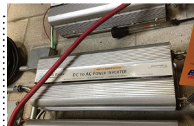
169B 10000 Watt 12 Volt Aims Power DC to AC Power inverter Installed in 2020
