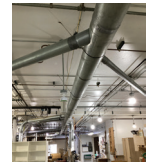
161 Dust Collection Pipe Throughout the Shop
