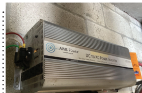
169C 10000 Watt 12 Volt Aims Power DC to AC Power inverter Installed in 2020
