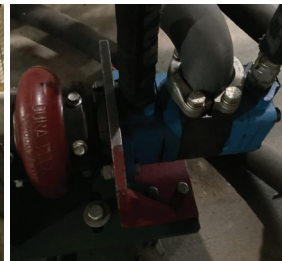
170 Complete Hydraulic Power System in The Engine Room, 7 Vickers Pumps, Oil Tank, Pipe and Shafts Tank Size Is 6 ft. Long x 3 ft. Wide x 42 In. high Vickers Pumps Listed Below 3520-25-9 2020-8-8 2010-8-4 2520-21-12 25V21 2020-8-8
