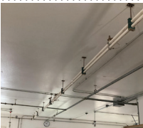
161A Humidifier setup Throughout the shop, Includes Water Storage Tank and Control Box
