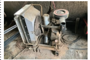
21 Rotorcomp model# NK-100up-V004 Air compressor serial# SC-210402
