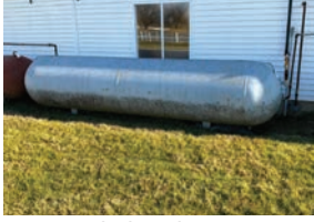
37 1000 Gal. Air Tank
