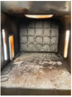
133 Finish Booth/build in booth -24" fan 230volt 1phase
