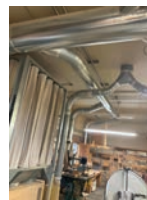
121 Newer duct work for entire woodshop, recently installed.
