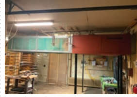
141 Air make up system / Powermatic model GA-115/476,928 BTU-115 volt, w/ air conditioner
