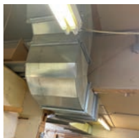
120 Ductwork for heat approx 82"
