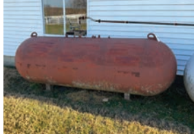
38 500 Gal. Air Tank
