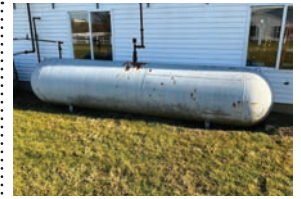
36 1000 Gal. Air Tank
