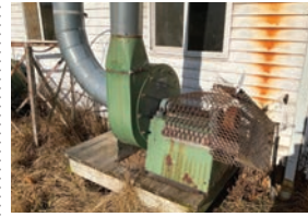
18A 24 inch blower, 10 inch inlet, 8 inch outlet
