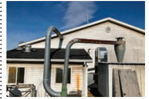
18B Cyclone and All pipe in attic
