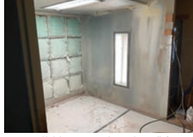
140 Build in Spray booth 24" fan
